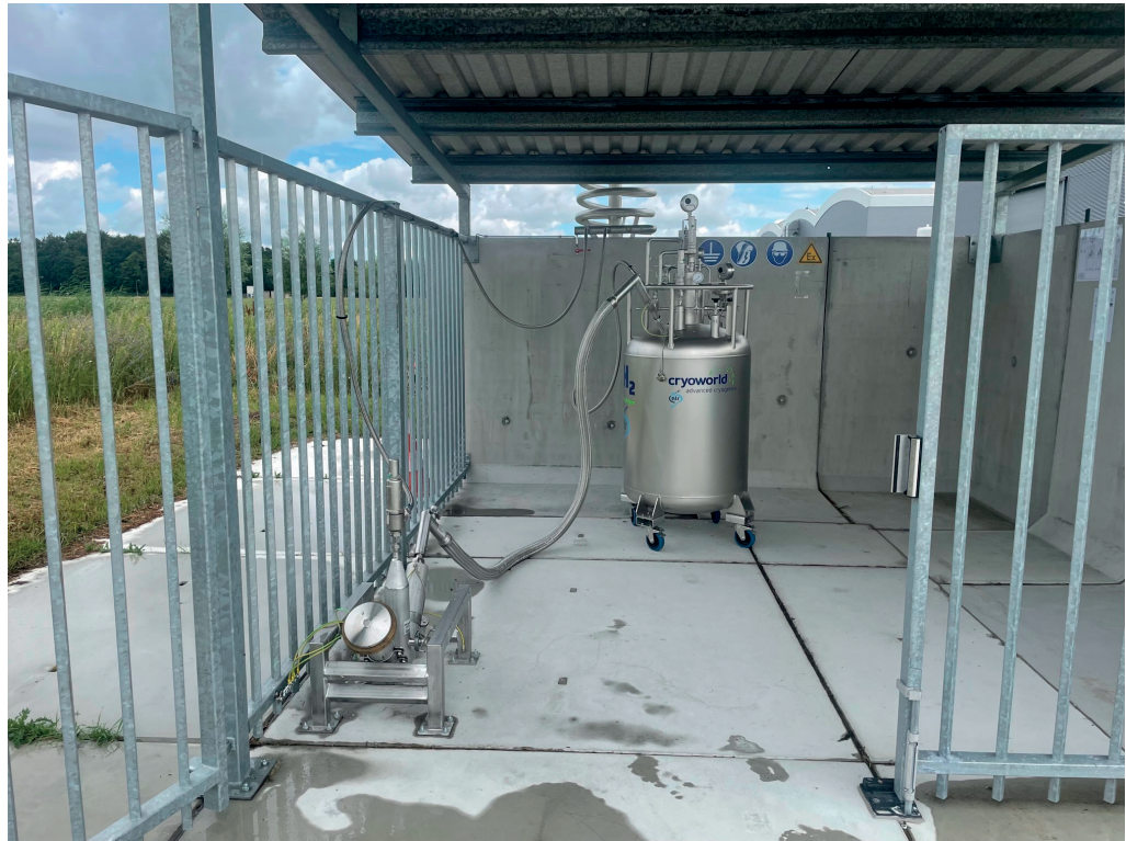
Figure 9 The LH 2 facility with the dewar (storage tank) and filling adapter Source: NLR
